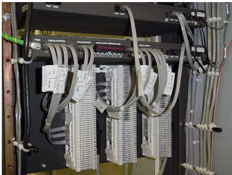
FIGURE 9-19 EXAMPLE OF CABLE LABELING
