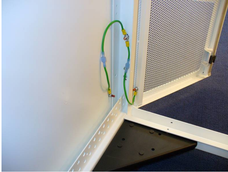
Figure 12 – Illustration of a bond connection from a cabinet to the cabinet door
